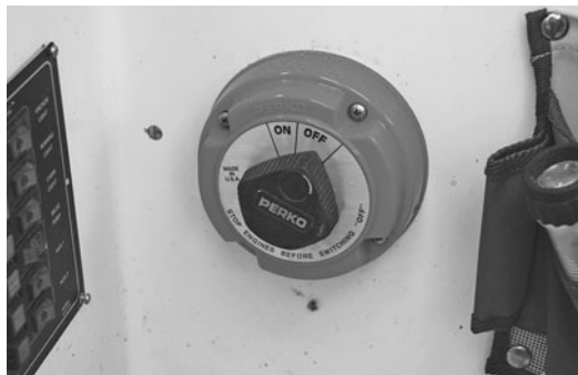
A heavy-duty battery switch for a single battery. This one does not include an alternator field disconnect, and could damage your alternator if switched while running your motor, if so equipped.
